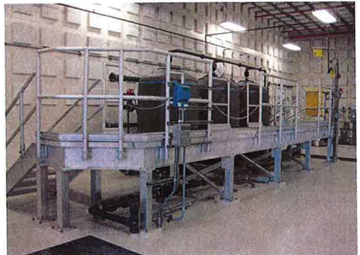
Calcite Contactors treat the water following reverse osmosis to add some calcium and alkalinity back into the pure water to make it less aggressive when in contact with metal plumbing.
