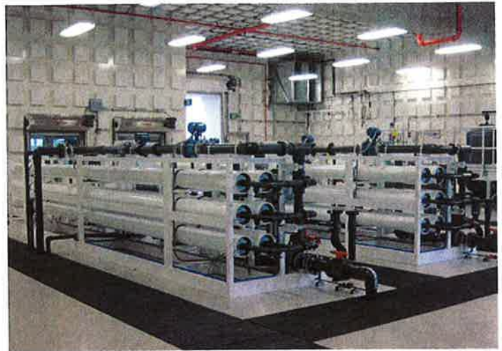
Two parallel Reverse Osmosis water treatment skids. Each skid can produce 200,000 gallons/day if operated 24 hours per day.
